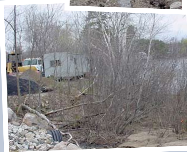
(bottom) State road construction and staging areas devastate water quality by not properly "phasing" projects or utilizing BMP'S (don't try this at home, it's more than a "technical" violation)
